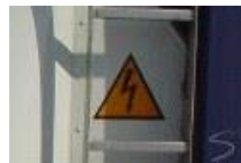
Figure 8.5 Overhead warning sign
